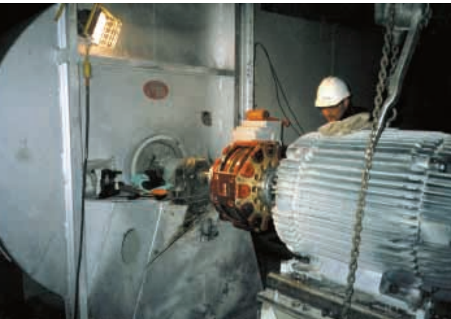
Magnetic ASD installation with a 125-hp 1,800 rpm motor and centrifugal fan. The ASD saves 155,000 kW-h of energy and $10,000 on maintenance costs annually.
