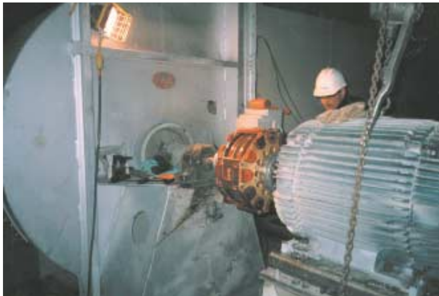
Figure 4: Magnetic ASD installation with 125 hp, 1800 rpm motor and centrifugal fan. The ASD saves 155,000 kWh of energy and $15,000 on maintenance costs annually.
