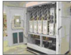
Figure 2. A large VFD system.
